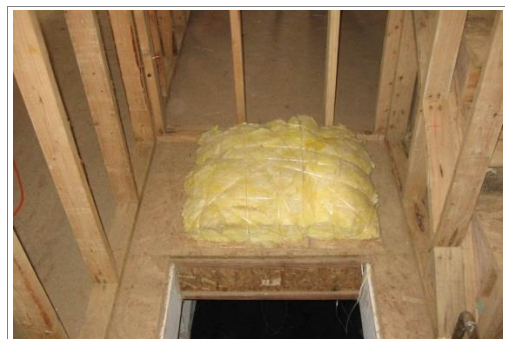
R402.2.4 Access Hatches and Doors Insulated crawl space access. The same method applies to attic access hatches.
